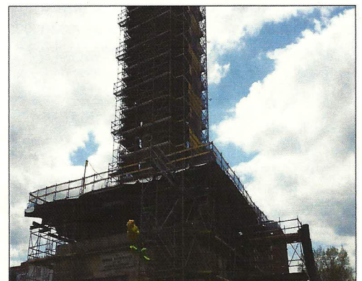
None of 'The Bulletin's' crack photographers could get a full shot of the Washington Monument; above, the base and portion of the statue. Completely wrapped in scaffolding, it'll take another year for completion.
